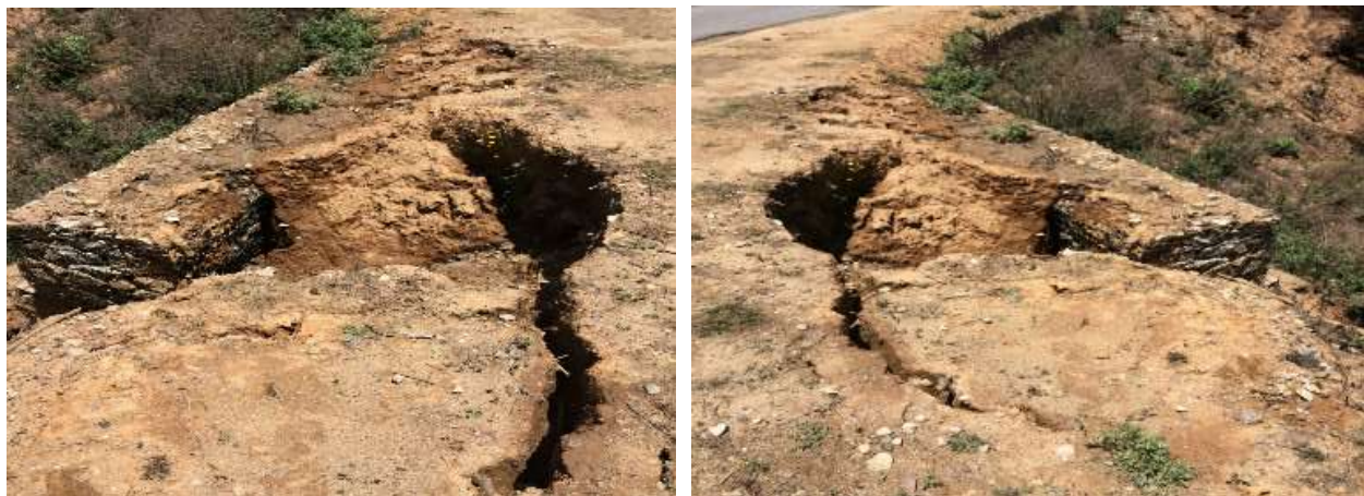
Fig: 7.2- Layers of gabion wall bulging outward
