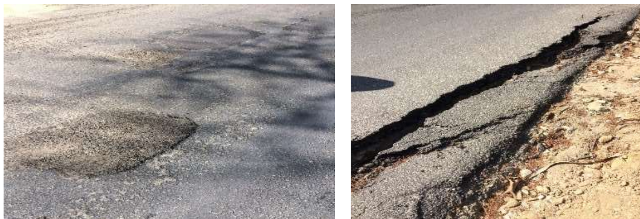
Fig: 5.4- Potholes not properly rectified and Depression of road at road edges
