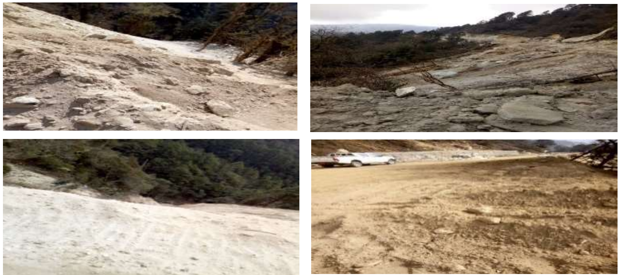
Fig: 2.17.8- Spoil materials dumped and freely rolled/pushed over the hill causing damaged to the environment
