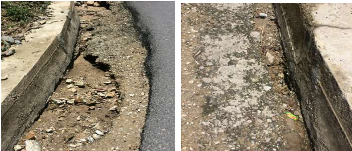
Fig: 7.1-Damaged L-drain
