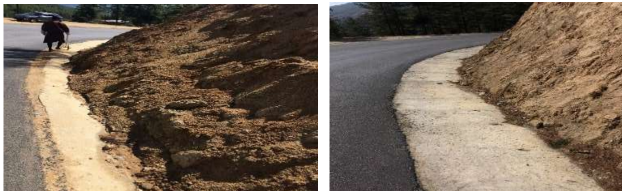
Fig: 3.3- L-Drain executed without plumb concreted
