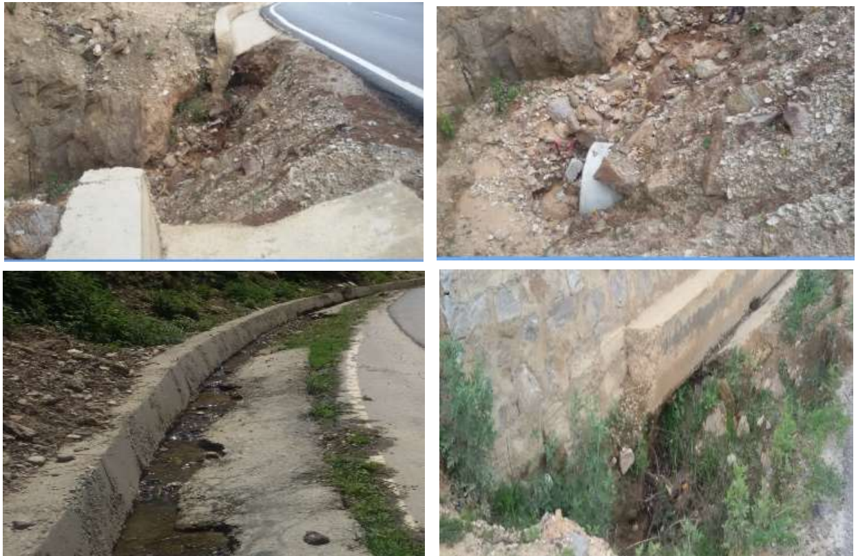
Damaged catchpit and drains
