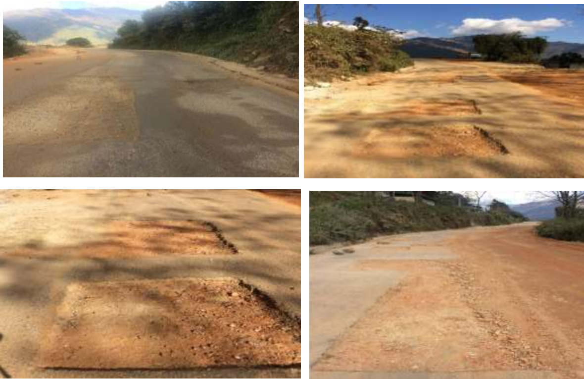
Fig 9.16(2)- Damages of ZeoCrete Pavement soon after execution of works
