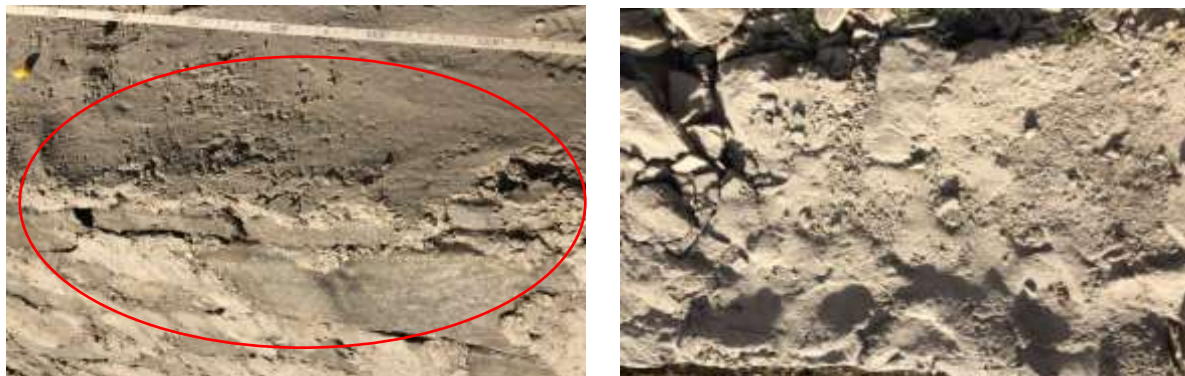
Fig: 3.3(a): Sub-standard R/wall without coping
