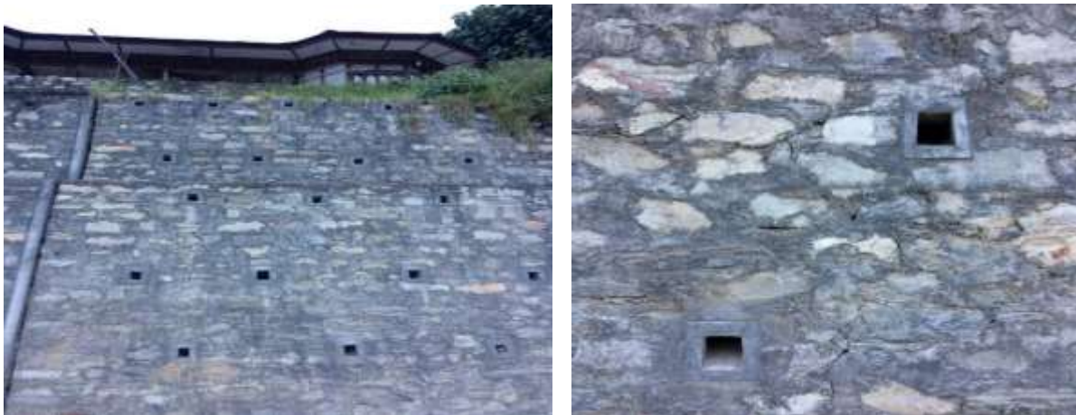
Fig: 4.6: Acceptance of defective RRM Walls and payments for works not executed
