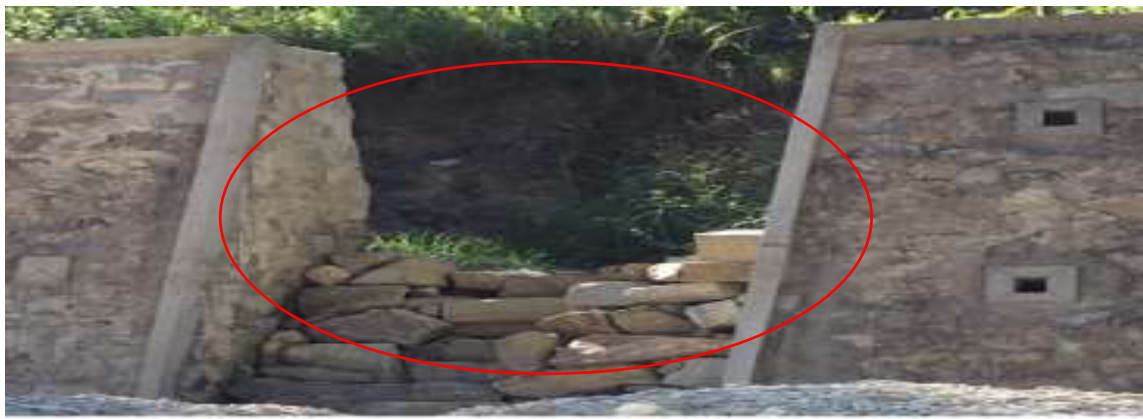
Para 23.4: Defective RRM steps
