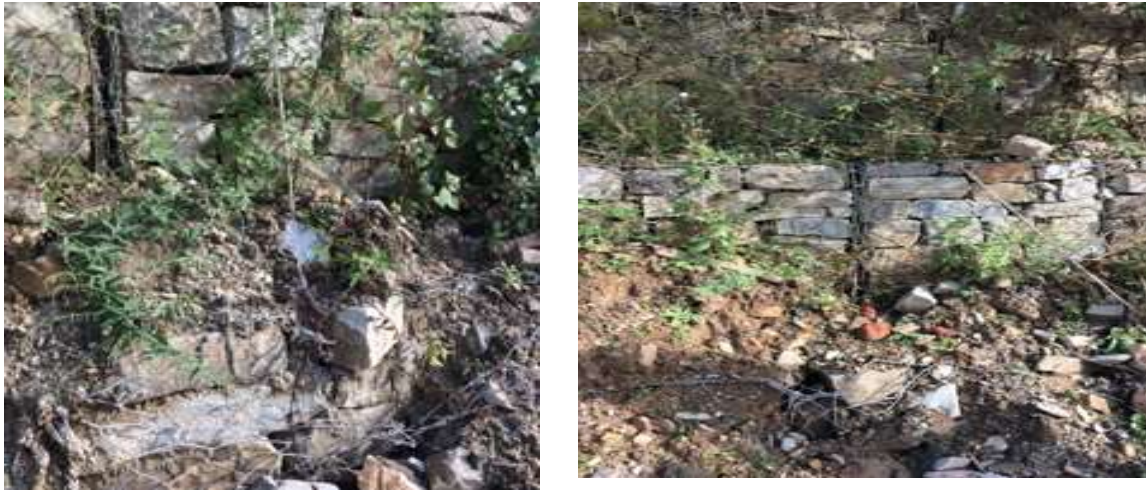
Fig: 23.3 Defective gabion wall with chain-link mesh torn off and gabion boxes bulging out
