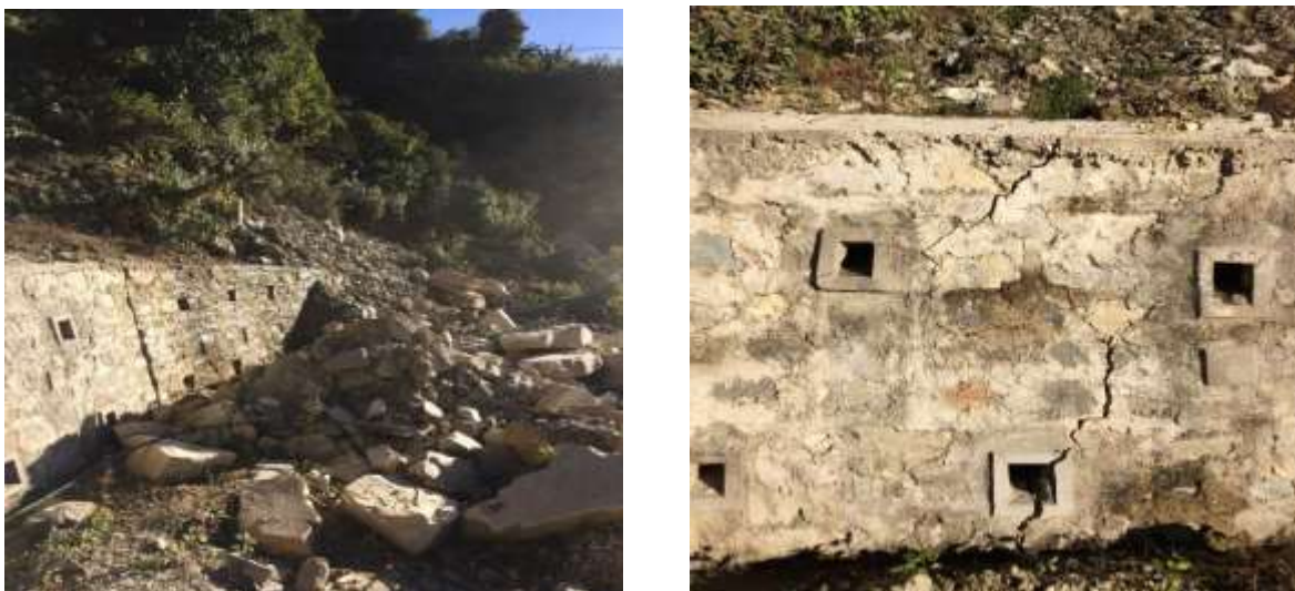
Fig: 4.6(a) Damaged RRM wall
