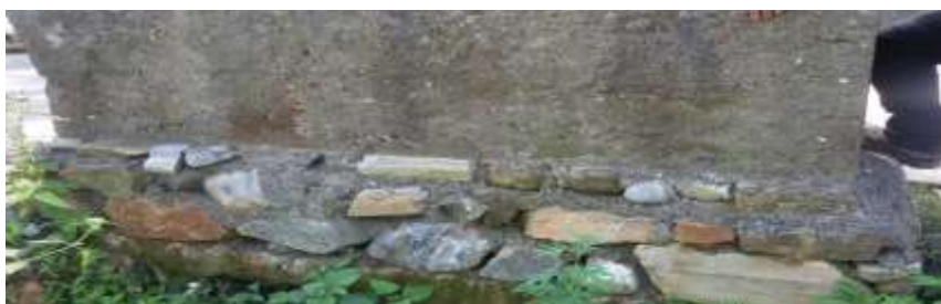
Fig: 23.2 Sub-standard construction of parapets & RRM above the slabs
