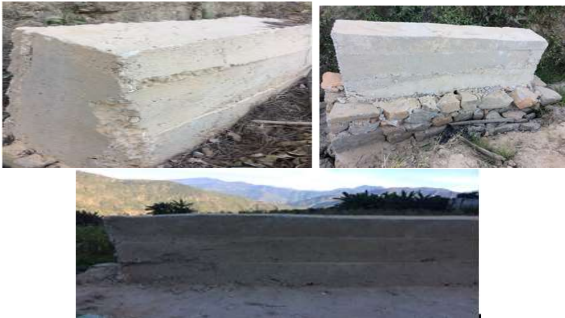
Fig: 21.3 Parapets with irregular shape and honey comb cracks
