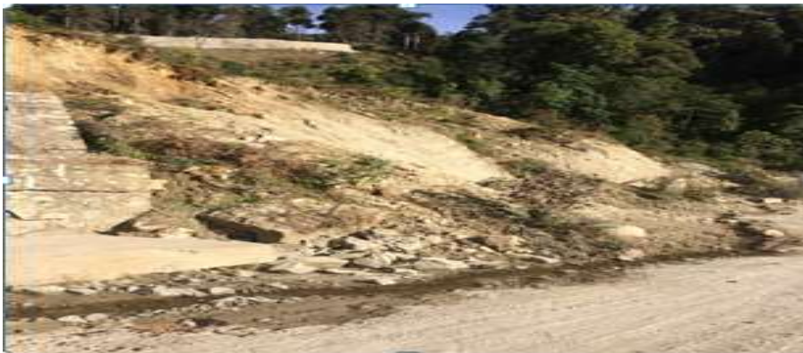
Fig: 3.3- B/Wall washed off by slide
