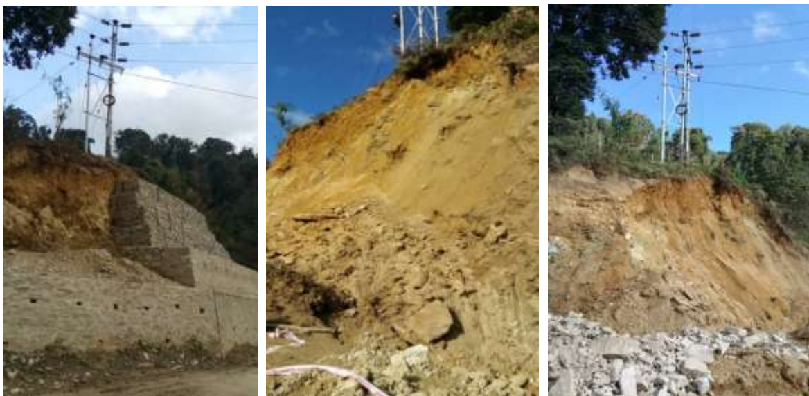
Fig:3.2- The above images shows the emergent need of restoration works to protect the transmission line
