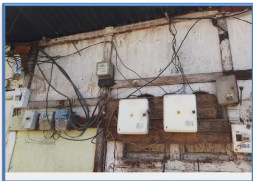
Open electricity meter box
