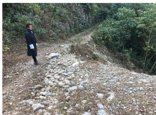
Samachen farm road abandoned due to unstable base, Darla, Chukha
