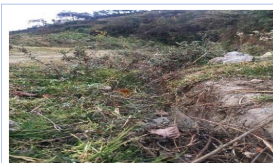
Bjabcho GC to Bjabchok Goenpa, Bjabcho, Chhukha, despite the formation of RUG, the farm road was covered by bushes.
