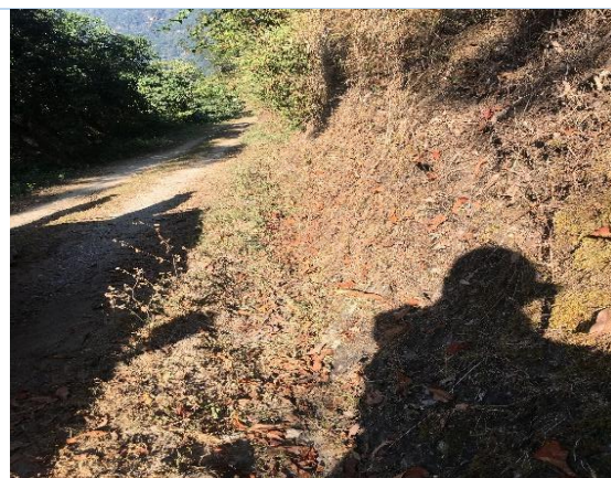
Damji farm road, Bongo, Chhukha. RUG conducted routine maintenance and the farm road was pliable all seasons.
