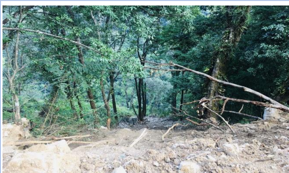
Excavated materials disposed off along the road Tsachhu approach road, Goenshari, Punakha.
