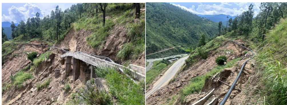
Figure 12: Irrigation channel and pipelines damaged by landslides
