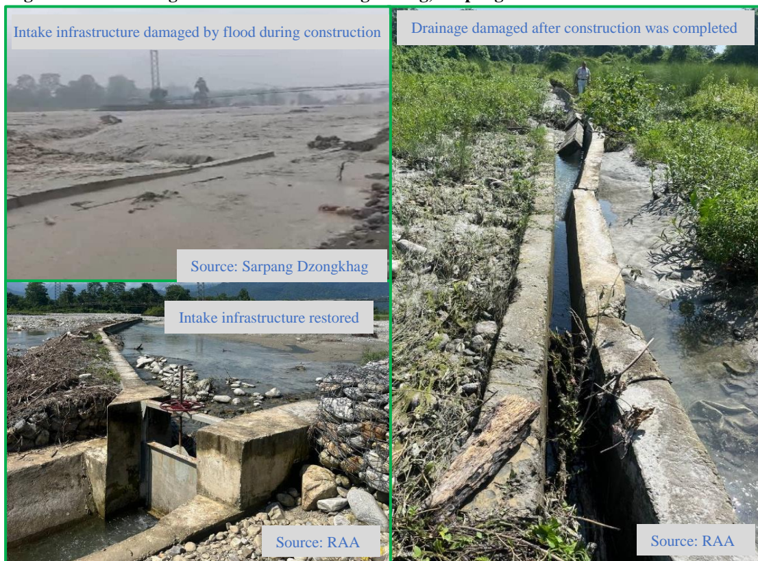
Figure 7: Gaden Irrigation Channel in Umling Gewog, Sarpang
