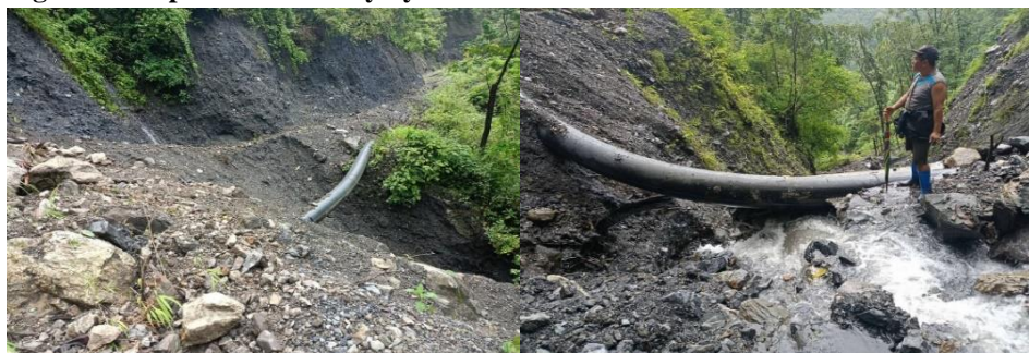
Figure 11: Pipes washed away by landslides
